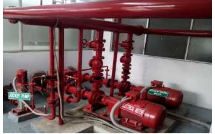
FIRE CONTROL ROOM 2
