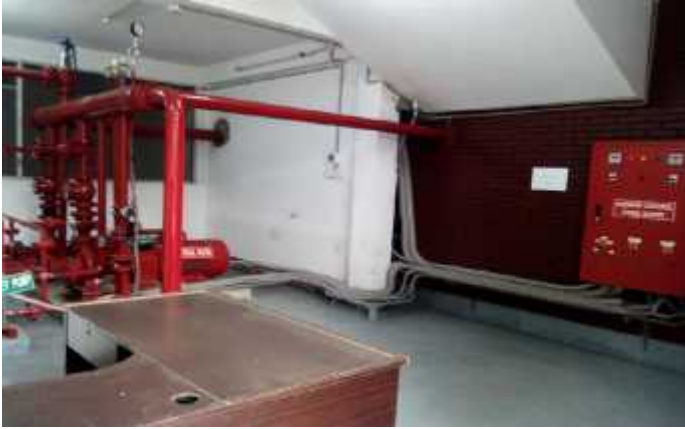
FIRE CONTROL ROOM 1
