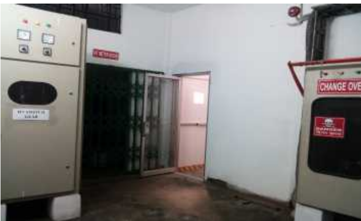
SUB- STATION ROOM 1
