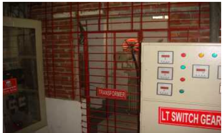
SUB- STATION ROOM 2
