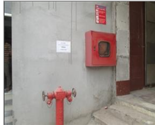
Photo of fire safety equipment Fire hydrant pillar and fire hose bucket.JPG
