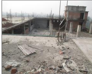
External photo(s) of the production unit(s) Construction work is going on (2).JPG
