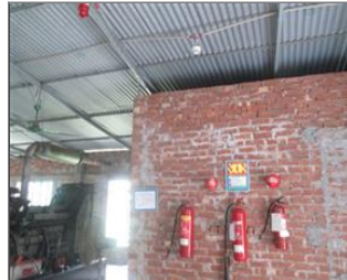
Photo of fire safety equipment Fire extinguisher.JPG
