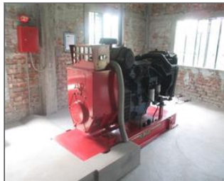
External photo(s) of the production unit(s) Generator.JPG
