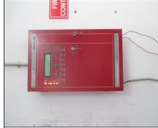
Photo of fire safety equipment Fire addressable panel.JPG
